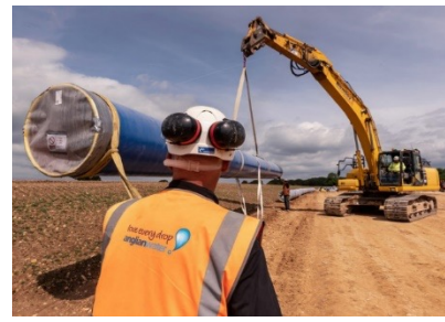
Delivery of the Strategic Pipeline Alliance (SPA), our biggest ever infrastructure development continues apace
